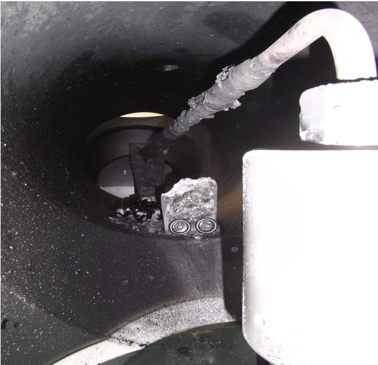
Figure 5: Cable Box Damage, showing the location of single phase fault
